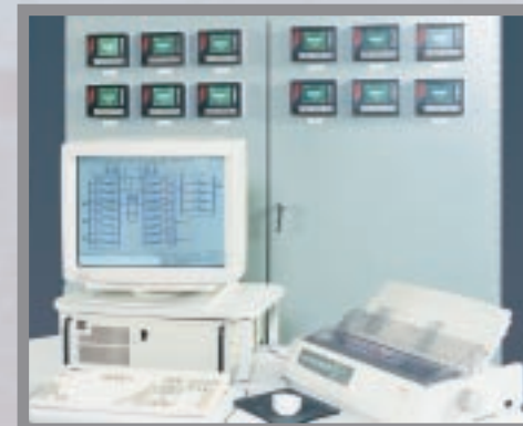
Advanced electronics control multiple meter runs.
