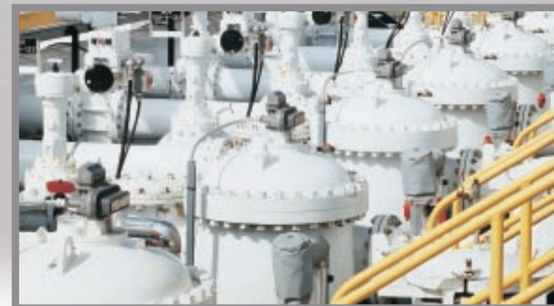
A pipeline metering system custom designed to optimize performance.
