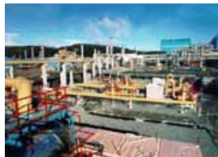
Complete Station, Statoil KUP, Norway
